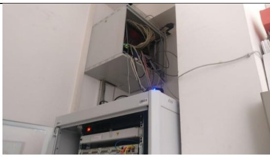
Figure 6-18 Centro stella in sala server
