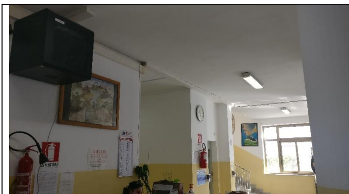
Figure 6-7 Switch piano terra rete Wifi
